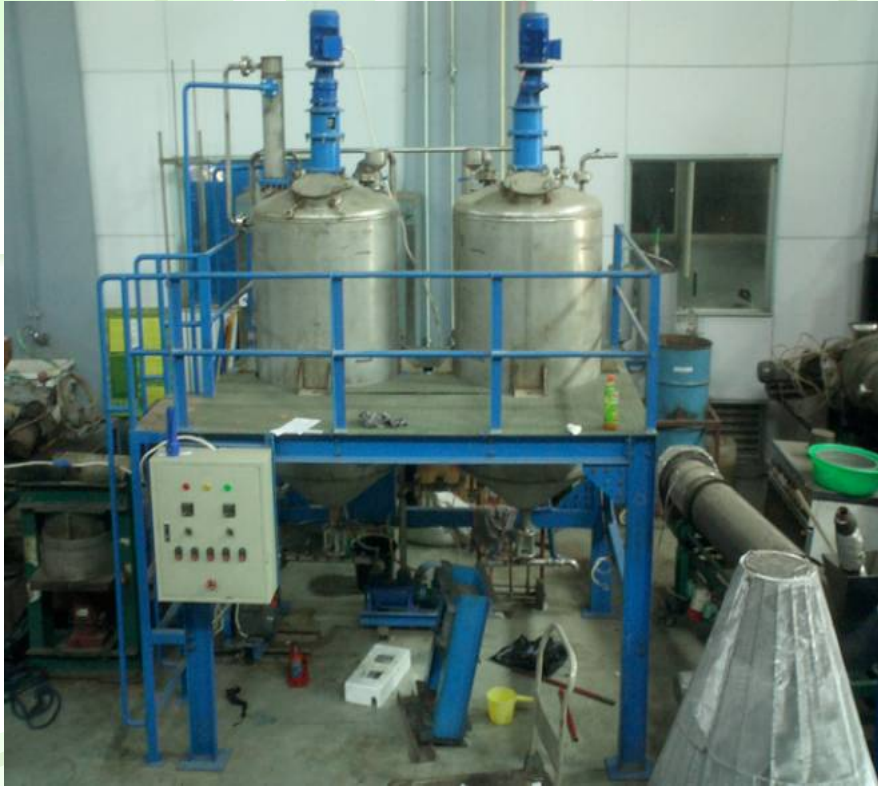
Recycling unit of waste-oil at Islamic School, Makassar (capacity 1 ton/day of 2 batch)
